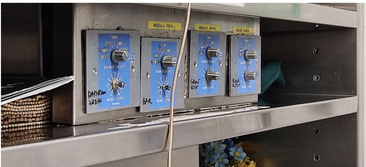
Figure 4: Cloud remote volume controls set operating level of the sound system in four zones in the premises
